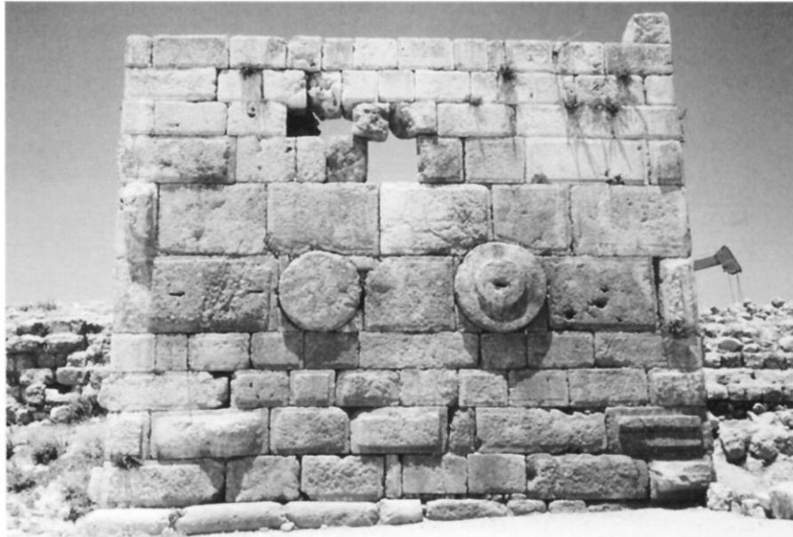
Fig. 2. Amman Citadel. South face of Ayyubid tower before restoration, showing the precarious condition of the slit window.
