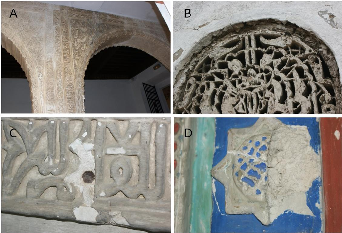
Fig. 4 Deterioration in RAS plasterwork: water seepage (A), direct action of rain (B), detachment after oxidation of the metallic element (C), disintegration of the material (D).
