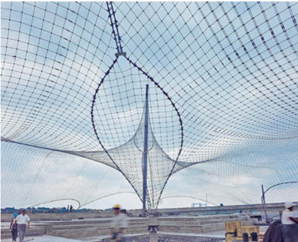
Fig. 7 West German Pavilion at the Expo '67 in Montreal under construction, Rolf Gutbrod and Frei Otto, 1967. The tensioned steel cable-net covers an area of 8,000 square meters by using a double curved geometry that is fixed at only 8 steel posts and surrounding ground anchors.
