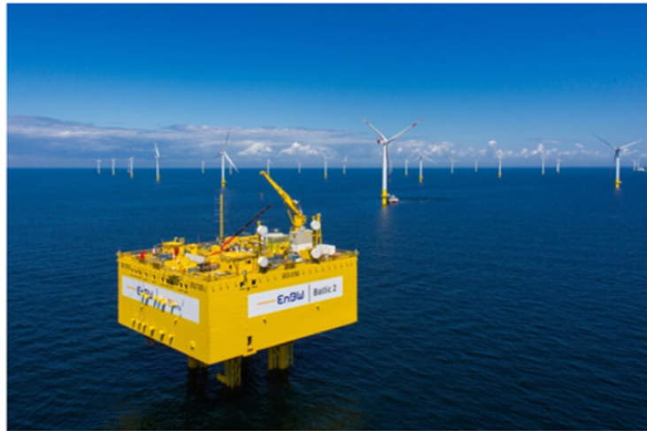
Alstom's GIS substations were installed on a platform at the Baltic Sea 2 offshore wind site. The platform was placed on a pre-installed jacket and brought out to the installation site where water depths reached 44 meters. The buoyant and self-erecting platform design enabled a high degree of flexibility and independency from crane ships for the transport and installation of the substation. The closed platform layout protects the electrical components from offshore conditions. (Credit: Alstom)
