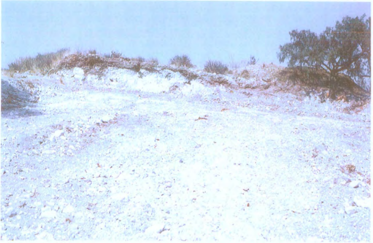
Plate 6.3 Breaking up of tepetate for the building of a terrace in Santa Maria Nativitas
