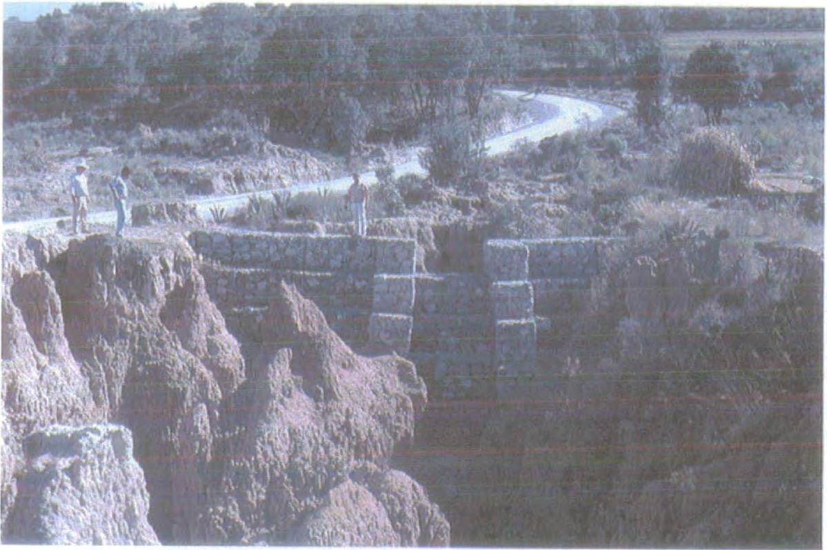
Plate 6.7 Gabion Dam constructed in a ravine in San Jeronimo Amanancla in the programme of Ecological restoration 1997
