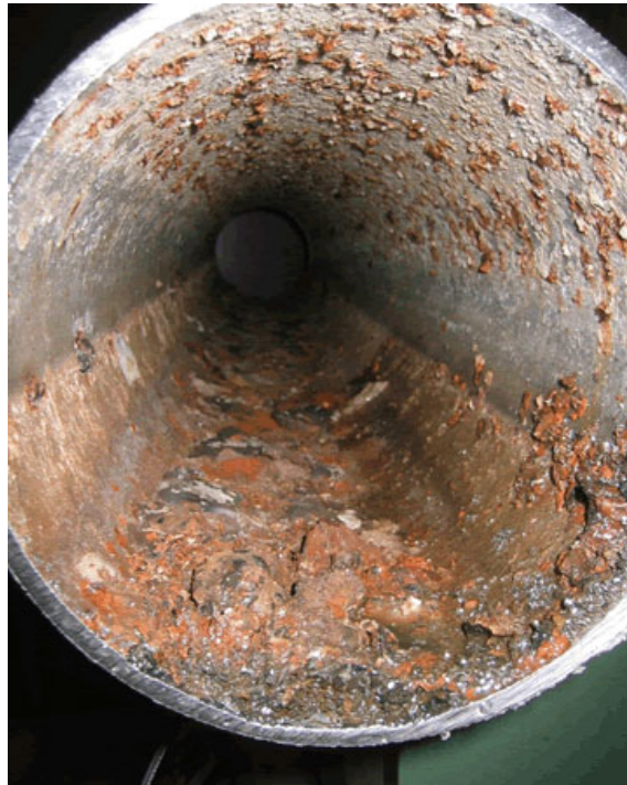
Figure 1.1: Internal corrosion of a typical pipework section
