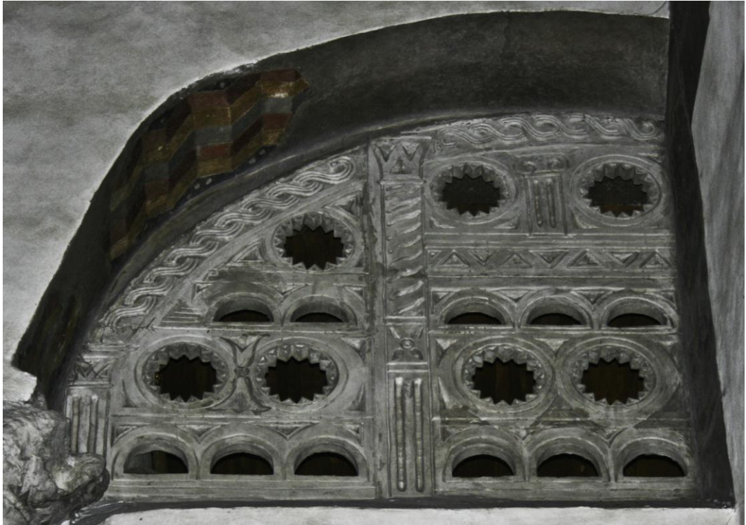
3.53 Pierced window insert, ninth century, S. Maria in Cosmedin, Rome (Photo: G. Dales)
