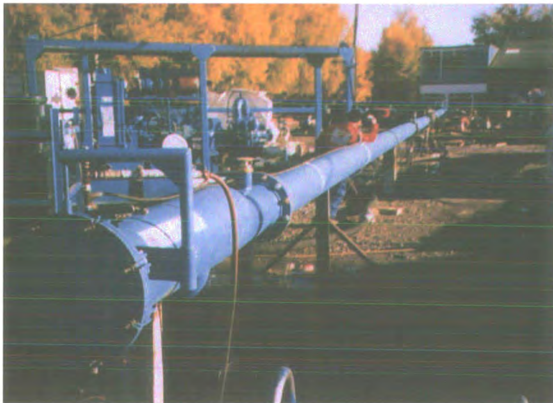
Figure 6.21. 12" Pipe loop at Pipeline Engineering's test facility
