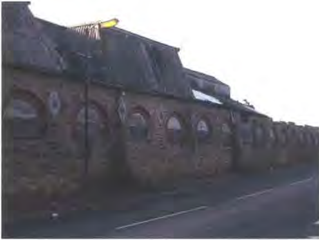
Fig. 117 This is the only remaining upstanding component of Spencer's Steelworks, Walbottle Road, currently used by a concrete manufacturer and recorded in 2004 (Tyne and Wear Museums) in advance of development (copyright author).
