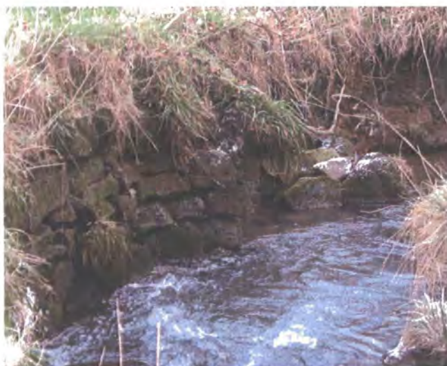
Figure 6.14: Example of a poorly maintained wall in Great Fryup Beck
