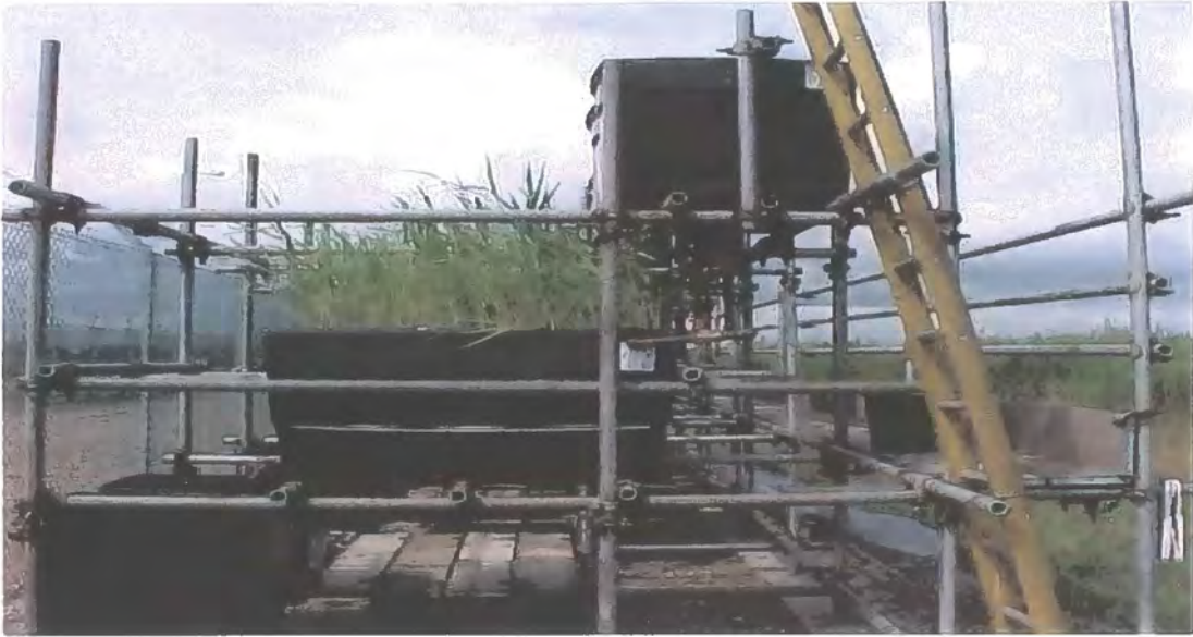
Plate 2.4. Side view of one complete test unit with test bed, header tank and receiver in place
