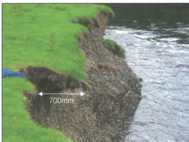
Figure 4.22: Considerable undercutting (indicated) at bank 3 following a rise in river levels, also note the oversteepened profile of the lower bank.
