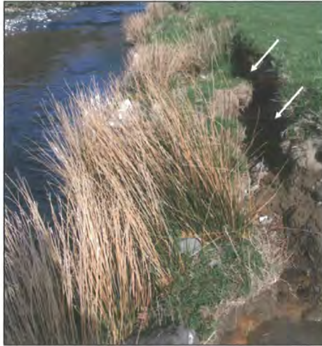
Figure 2.16: Shallow slip failure on the river bank of St. John's Beck, St. John's-in-the-Vale, Cumbria. The failed block has not been further eroded and it remains well vegetated. An obvious tension crack (indicated by the white arrows) is situated between the failed block and the retreated bank face.
