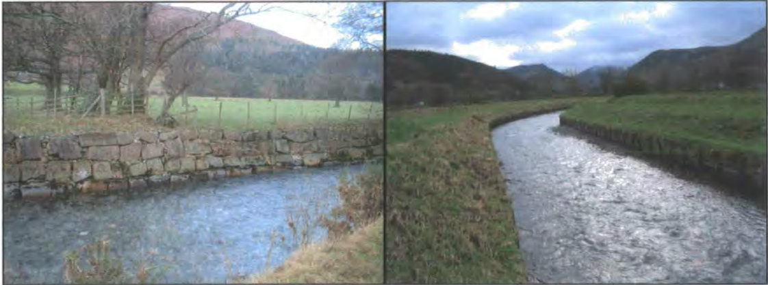
Figure 2.5: Channel regulation on Newlands Beck, showing channel straightening and bank heightening and reinforcement using (left) boulder revetments (NY 238 221) and (right) wooden revetments at Newlands Bridge (NY 240 263).
