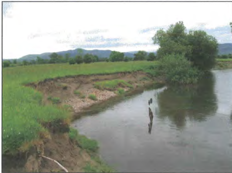
Figure 2.6: A line of ruinous wooden revetments in the River Derwent's channel at erosion study bank 2 near Low Stock Bridge (NY 237 266), showing obvious retreat and erosion of the bank back from the revetments.
