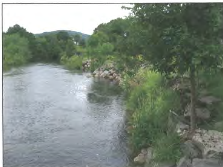
Figure 4.42: Large stone revetment in the form of a raised embankment on the east bank of the River Derwent to the north of the A66 bridge (NY 250 241, looking downstream).
