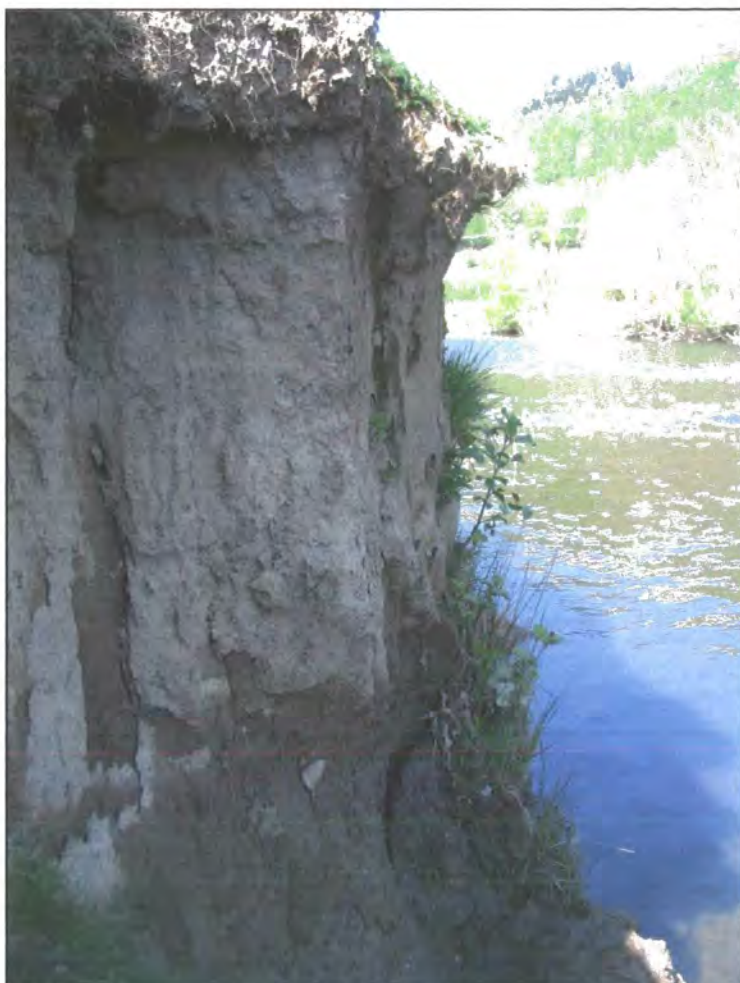
Figure 4.36: Desiccated river bank face downstream of Low Stock Bridge at NY 235 269, showing the moisture contrast between the (dry) upper and lower bank.
