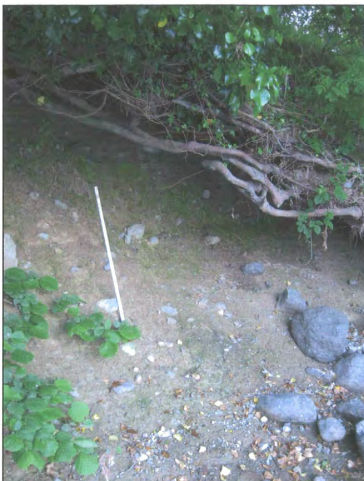
Figure 4.29: High (3.5 m) but presently stable river bank near Portinscale (NY 252 238), with metre ruler for scale. The dense vegetation roots at the overhang and the highly cohesive till on the lower, exposed bank face have prevented active erosion of this bank.
