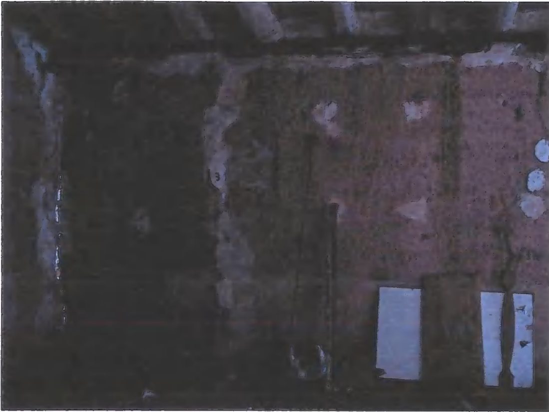
Figure B.13 Cracks 1 to 4. East wall internal. Roof level of north east tower
