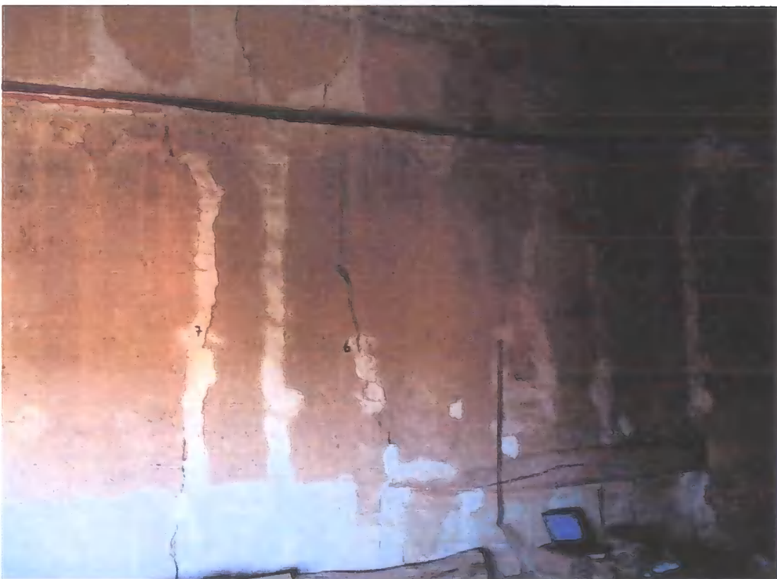
Figure B.14 Cracks 5 to 7 and timber repair. West wall internal. Roof level of north east tower
