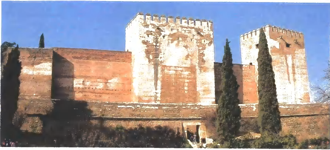
Figure C.46 Gr1a Cracked tower ( Torre Quebrada ) (right) and Keep ( Torre Homenaje ) (centre)
