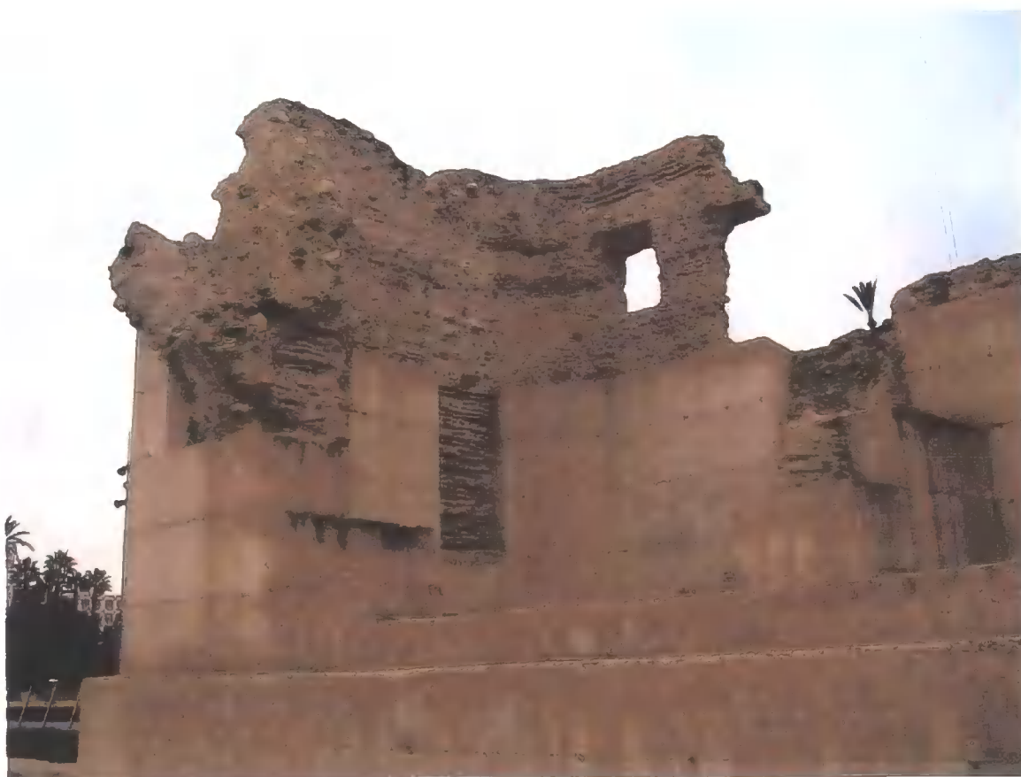
Figure C.41 E13 Elche consolidated ruins, note concrete repairs
