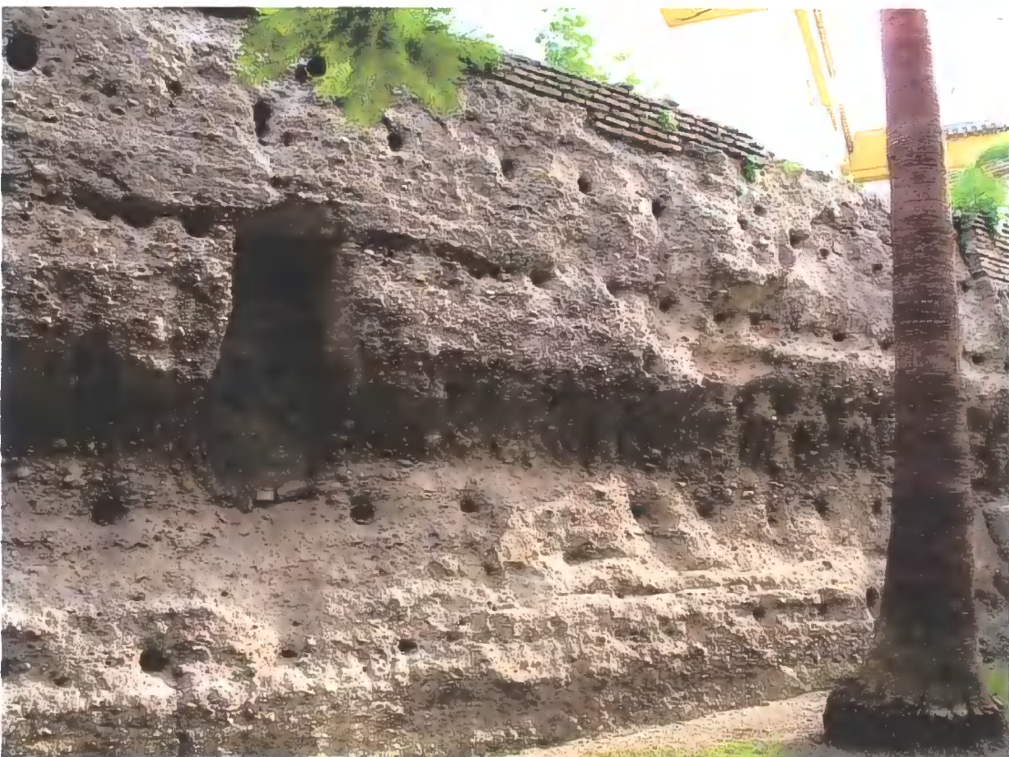
Figure C.77 Pa2 Heavily eroded section, Palma del Rio
