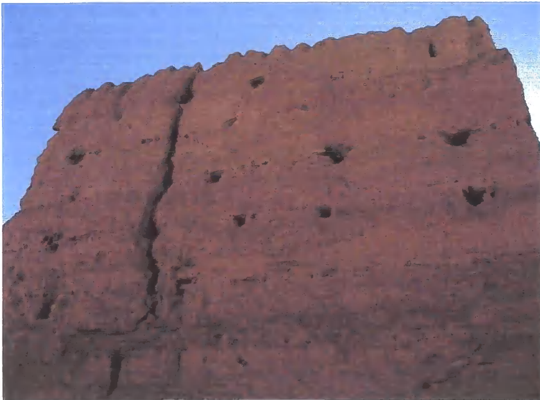
Figure D.20 Bg1b Basgo crack stitch photograph
