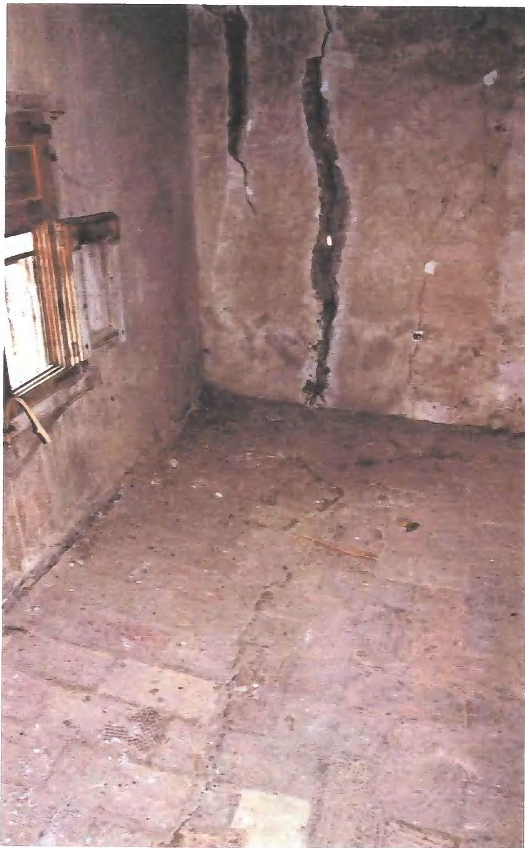
Figure B.15 Cracks 9 (left) and 10 (right), and gap between floor and wall. First floor. East wall of north east tower
