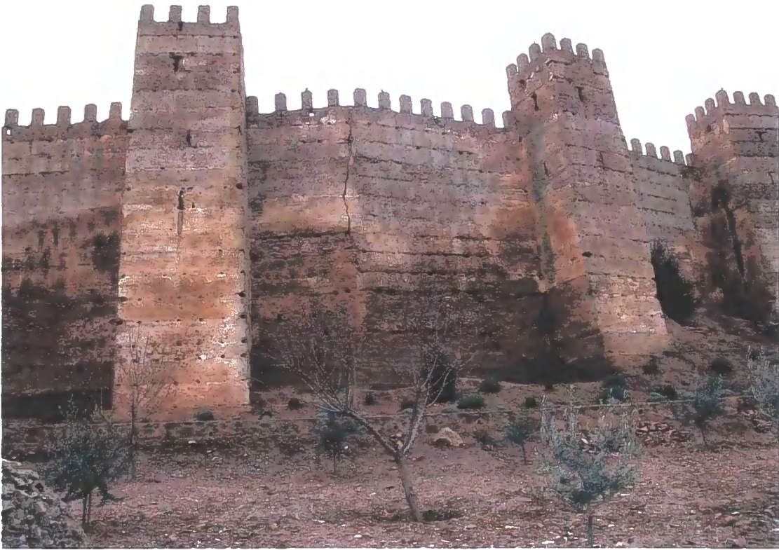
Figure C.18 Bale Crack between towers 2 and 3, note cement repair at base
