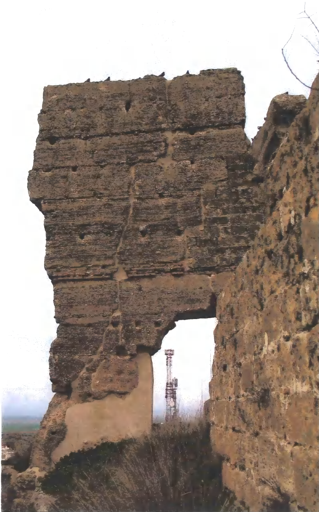
Figure C.24 Ca1a Earthquake damaged tower, Carmona. Constructed 1502
