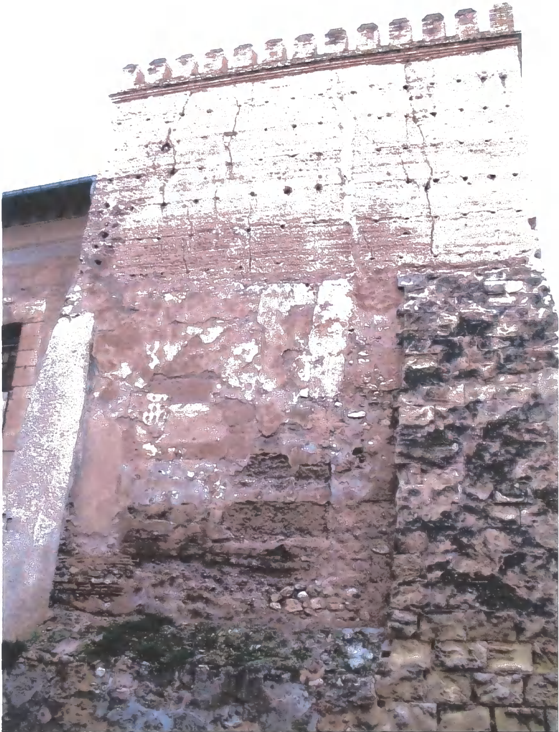
Figure C.43 El2 Elche Town Hall, situated at the end of the church. Once a mosque, there is a large Muslim Crescent on the roof
