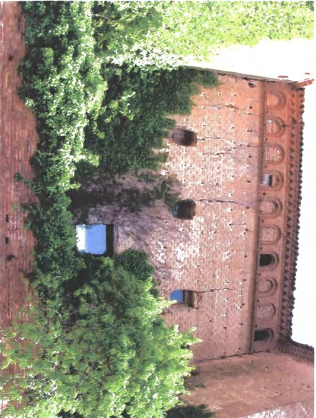
Figure B.11 Central section of Ambel preceptory. Cracks suggest settlement of north east tower (left)
