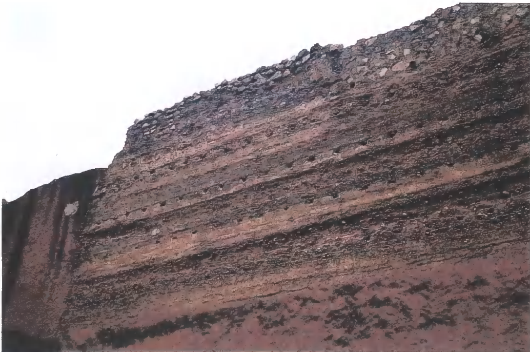
Figure C.73 No3 Eroded north face of curtain wall
