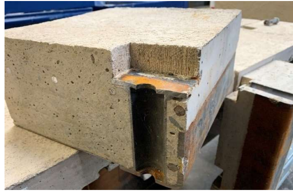
Figure 2 Photo shows a cross-sectional view of a prefabricated concrete slab, embedded steel tube with welded plates
