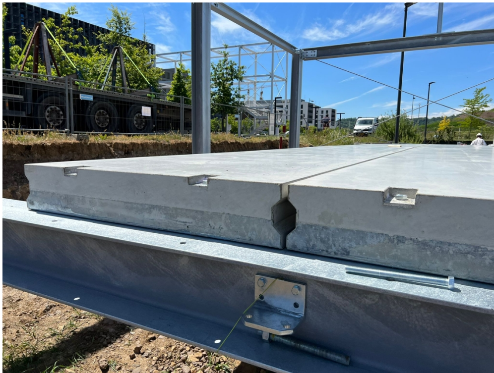
Figure 7 Photo illustrates the grids for bolts between the concrete slab and its supporting steel beam
