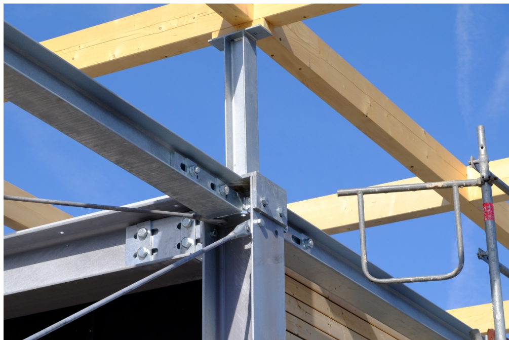
Figure 8 Photo shows complex joints where members meet in multiple directions 1727x1151mm (72 x 72 DPI)
