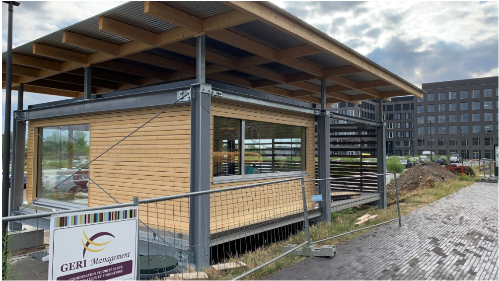
Figure 4 Photo shows the axis of columns following a proposed standard grid 1422x800mm (72 x 72 DPI)
