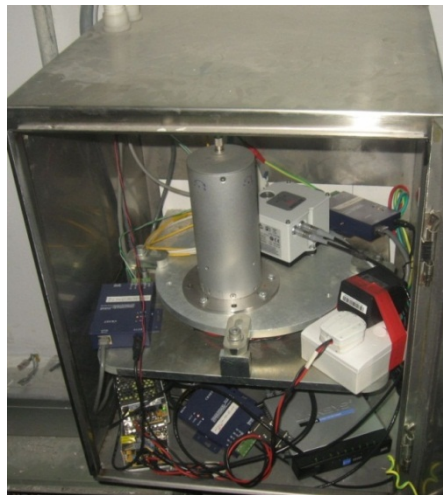
Fig. 6 Inclinometer installed on the structure
