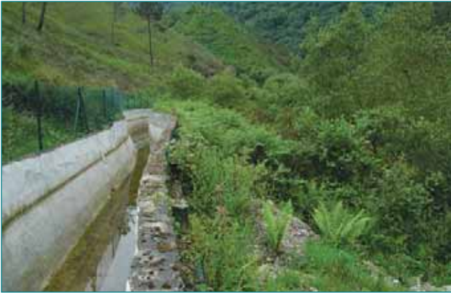
Feeder channel for small-scale hydro-electric generation; Picos-18.
