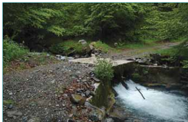
A double-culvert crossing point – the only modification along the 2km of Picos-13 to 16.
