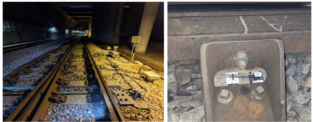
Figure 11. Site 3: swing-nose crossing and example of the low-cost accelerometer installed on the bearers.
