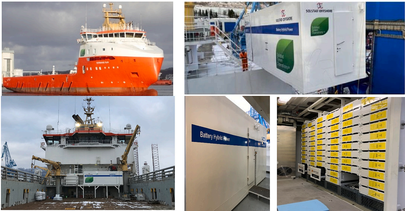
Fig. 1. The 500 kWh BESS retrofitted onto NS in 2018.
