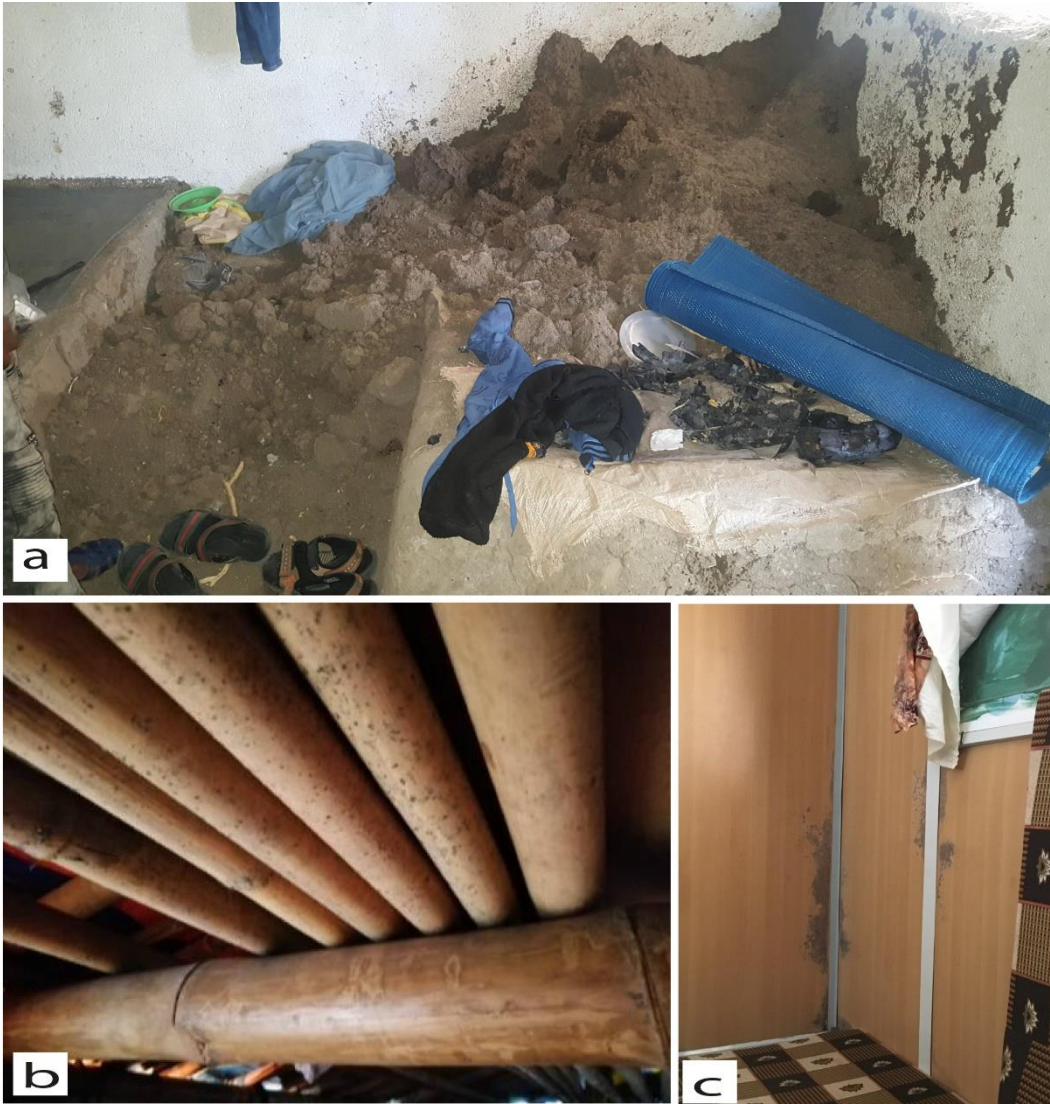
Figure 15: (a): Termite mounds inside a shelter, Ethiopia (b): termite-infested bamboo shelter, Bangladesh; (c): Mould growth on MDF inner surfaces in Zaatari camp, Jordan. Photos credits: authors.
