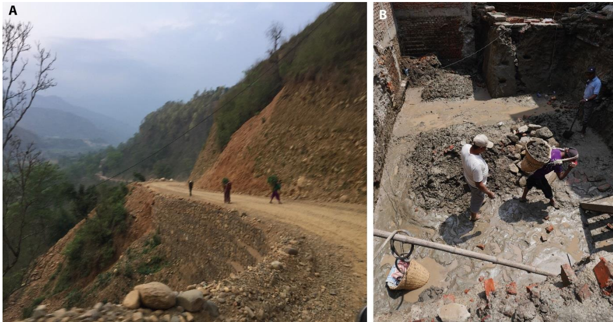
Figure 7. (A) The road that accesses communities on the Salyantar terrace is cut into a steep escarpment that is vulnerable to instability during monsoon rains. (B) Excavation in silts and fine sands with a sump pump, for building foundations in Bhaktapur in April 2018. Evidence for liquefaction below the feet of the construction workers. Local people reported that this stage of reconstruction is not possible during the monsoon.
