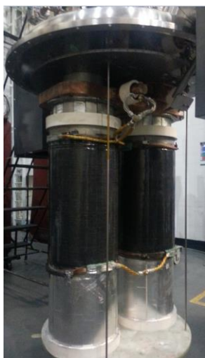
Figure 8: 11 kV SFCL coil using MgB_2 superconductor at University of Manchester
