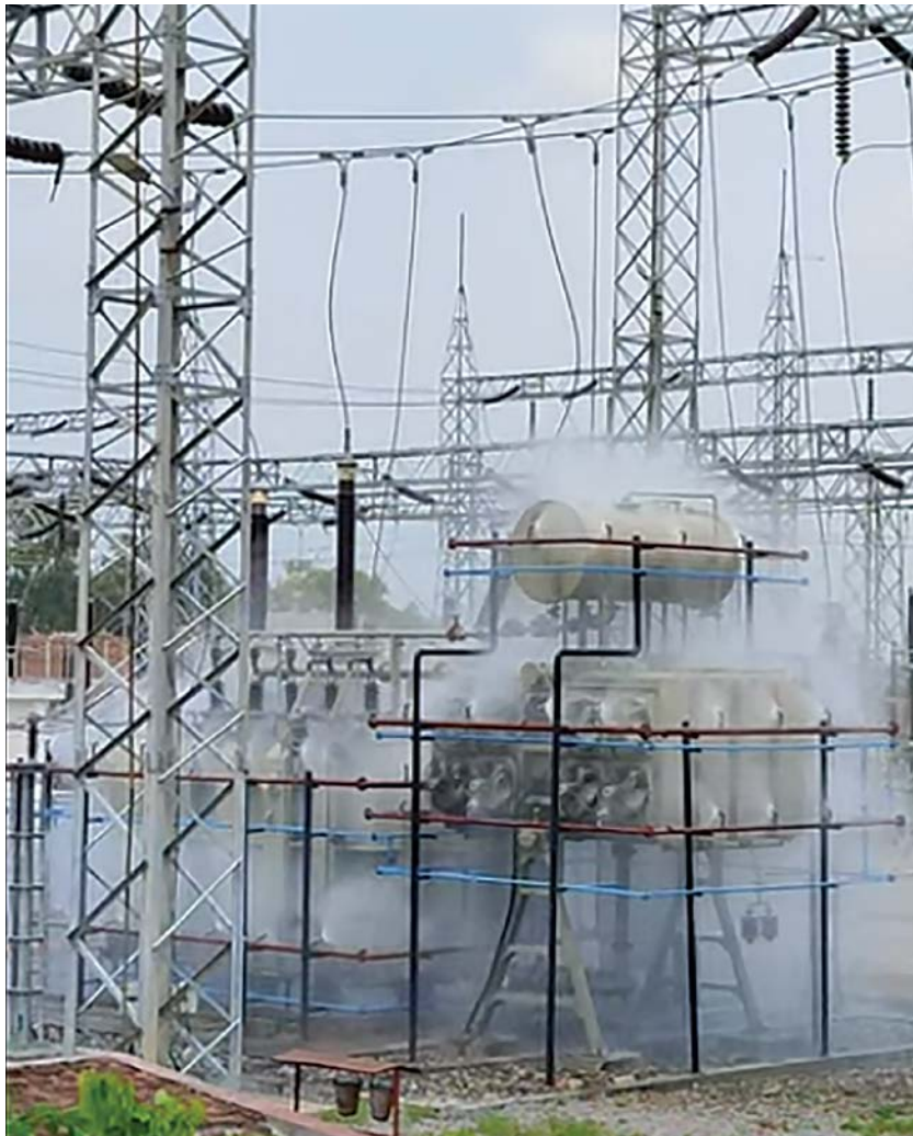
Figure 9. Automatic MultiFyre system
