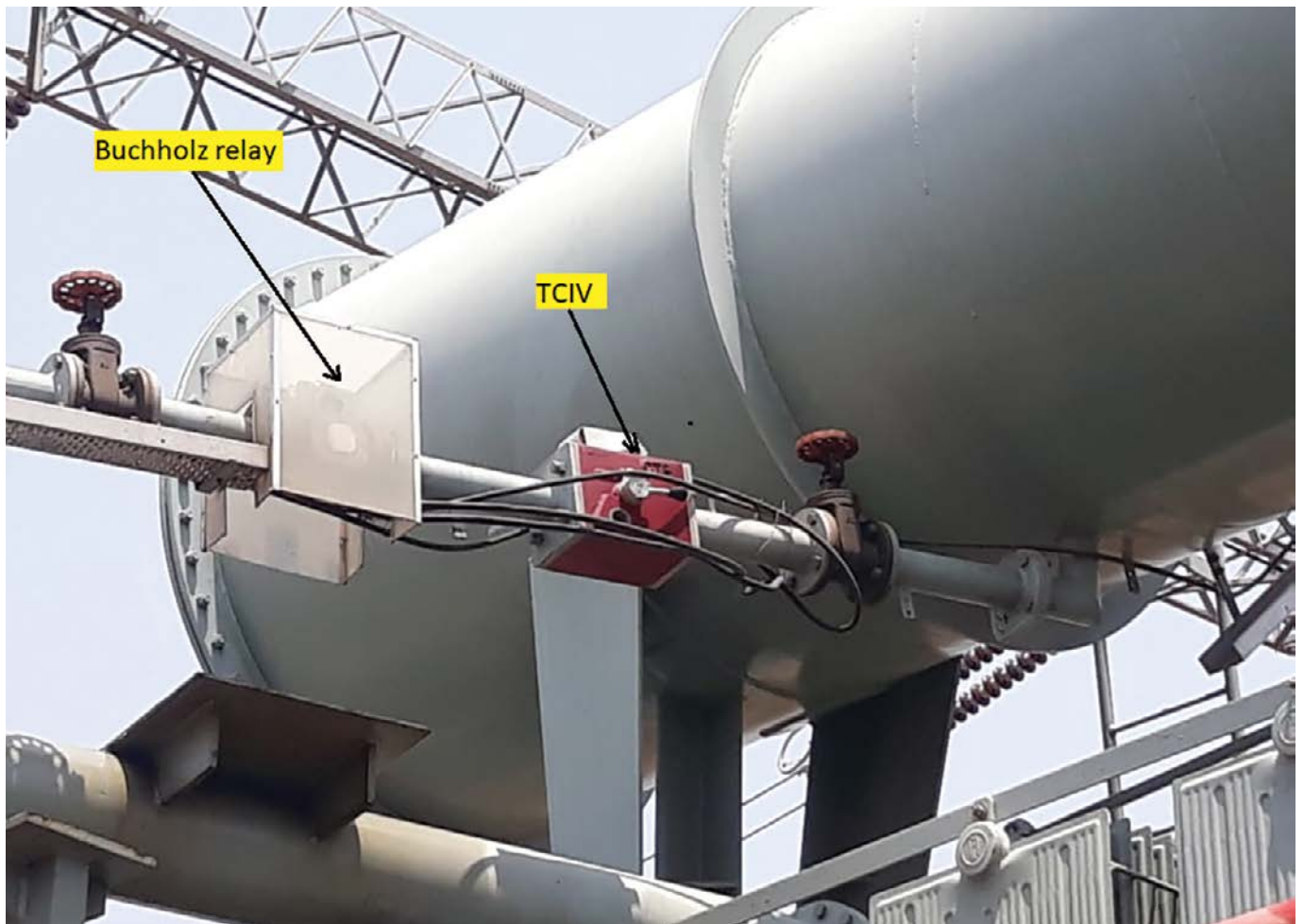
Figure 8A. Showing a Buchholz relay (with acrylic cover to protect against rainfall) and TCIV (Transformer Conservator Isolation Valve)
