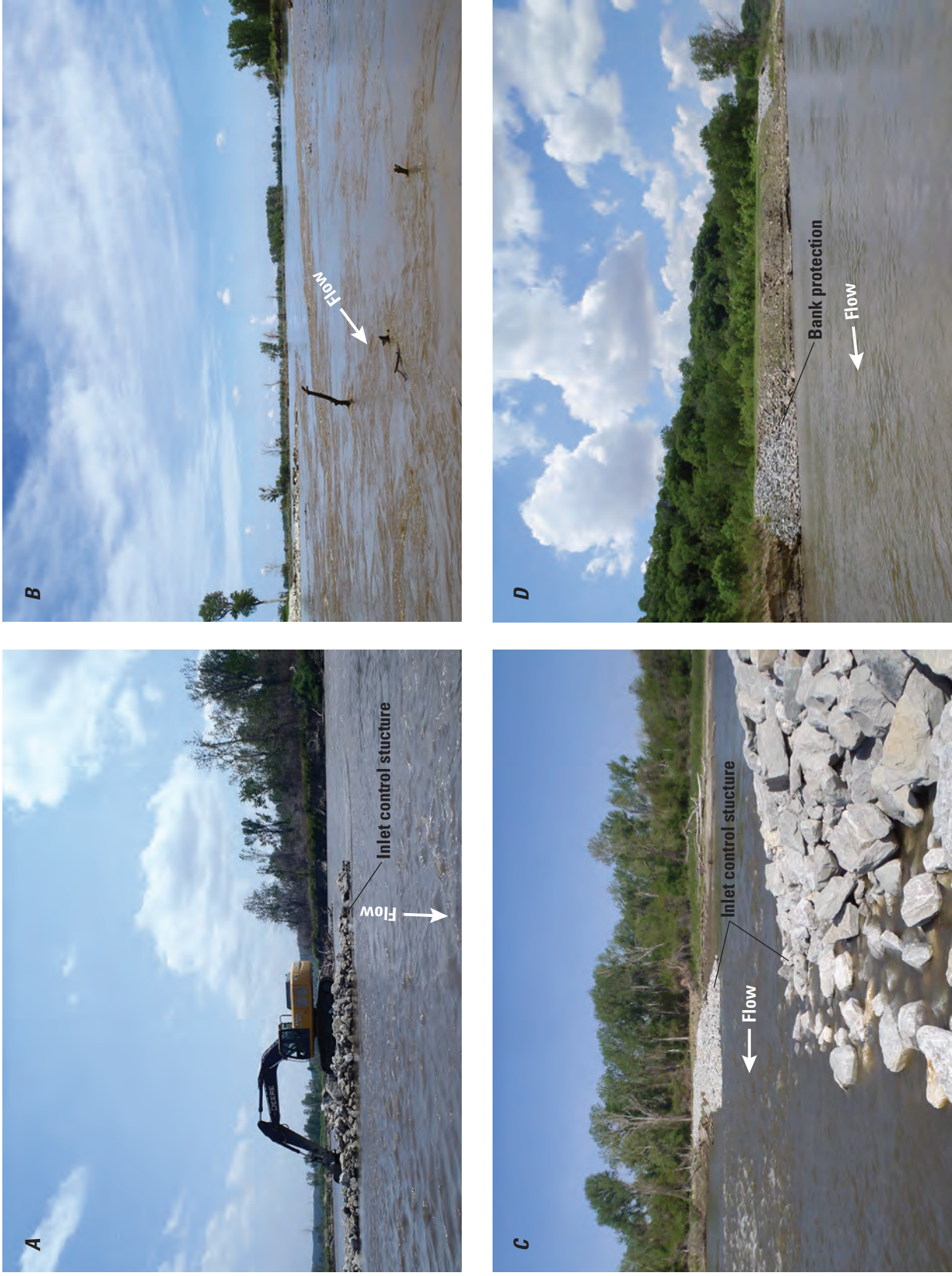
Figure 2. Control structures at Missouri River chutes, 2011–13. A , Construction of a new inlet control structure at Deroin chute, 2013. B , Turbulent water around the inlet control structure and snags at Lower Hamburg chute, 2014. C , New control structure within Lower Hamburg chute, 2014. D , Limited bank protection on an eroded bank at Tobacco chute, 2014.
