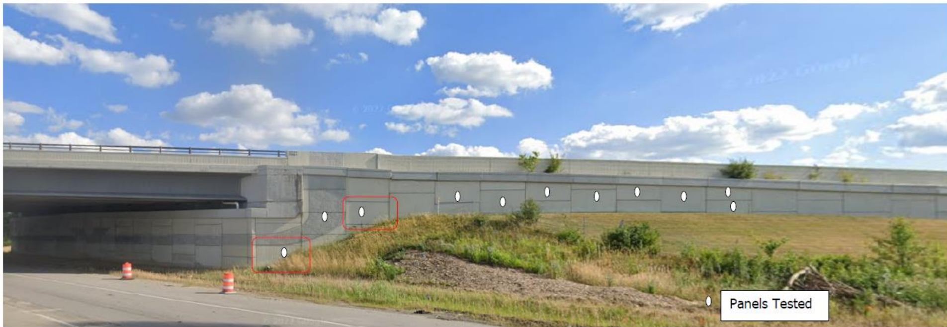
Image showing the wing wall and panels with air gap GPR signatures (red).
