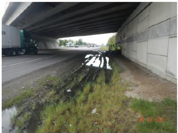
Abutment 1: Standing water due to inadequate drainage
