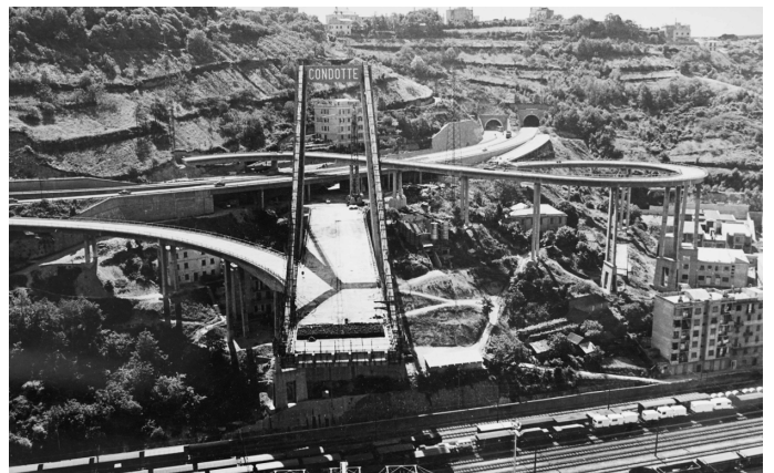
Figure 1. Aerial view of the helical ramp under construction / Vista aerea della rampa elicoidale in costruzione
