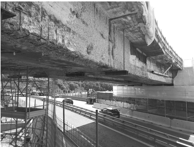
Figure 9. Interventions on buffer span between P28 and P29 piles/ Interventi su campata tampono tra pile P28 e P29.
