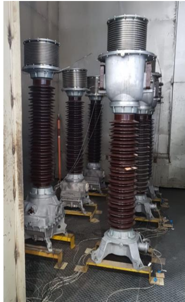
Figure 30 – Test circuit arrangement inside oven.
