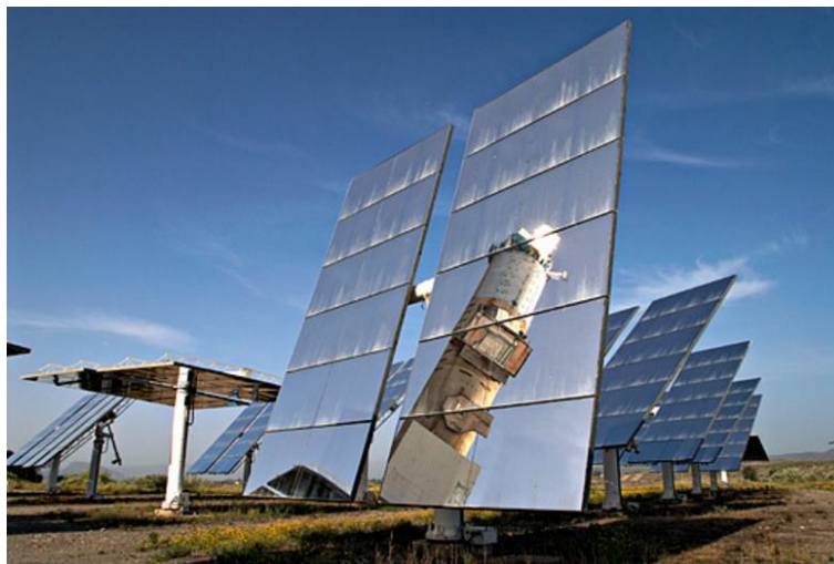
Fig. 53 Colector Heliostato Sanlúcar 120
