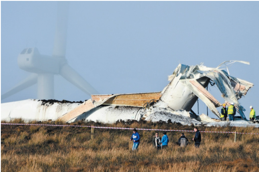
Fig. 1.3. Disintegration of a wind turbine in Ireland on 2 January 2015 due to a fault in turbine control system [Reproduced with permission from [Andrew Kusiak, “Renewables: Share data on wind energy,” Nature , vol. 529, no. 7584, pp. 19-21, Jan. 2, 2016.] Copyright 2016, Nature Publishing Group], [5, 6].
