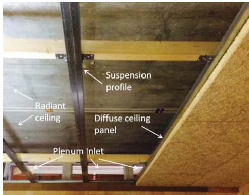
Fig.4. Diffuse ceiling panels and radiant ceiling
