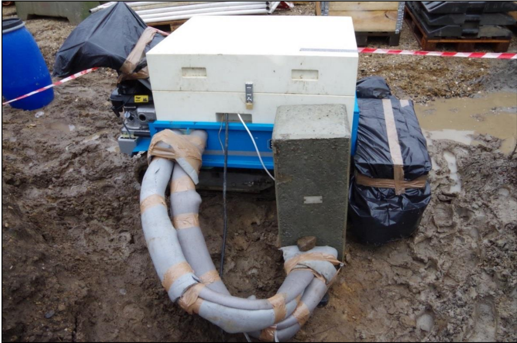
Figure 17: Ongoing TRT of the 18 m long EP3 at Langmarksvej. Inlet- and outlet pipes are insulated to prevent disturbances from ambient temperature conditions. The adjacent box, covered by black plastic bags, contains the computer and the modules to log the temperature data from the underground Pt100 TSA.
