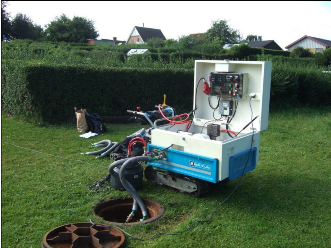
Figure 13: Ongoing TRT at the 18 m deep BHE at Langmarksvej. Inlet- and outlet pipes are insulated to prevent disturbances from ambient temperature conditions.
