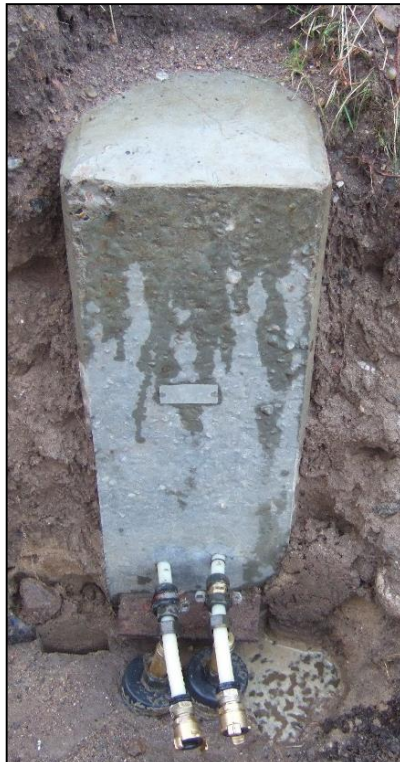
Figure 14: A single EP at the Langmarksvej test site prior to connecting the TRT equipment.
