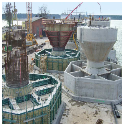
Figure 1.8: Heavy weight foundations for the Horns Nysted II offshore wind farm. (Bilfinger Construction 2015)
