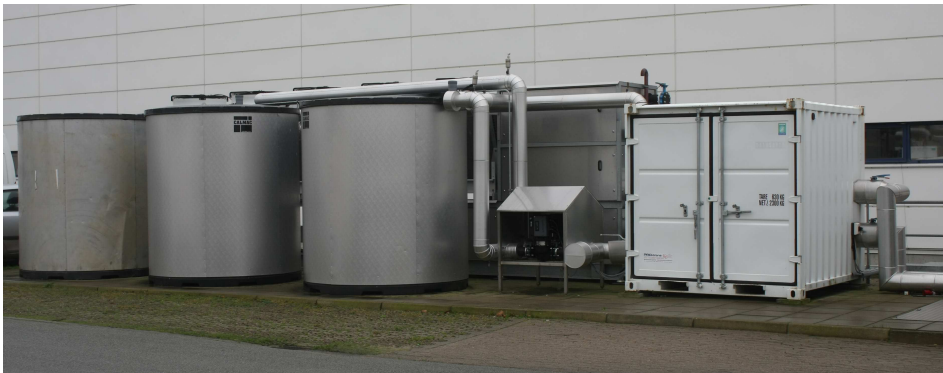
Figure 6.8: Grundfos chiller with the ice storages
