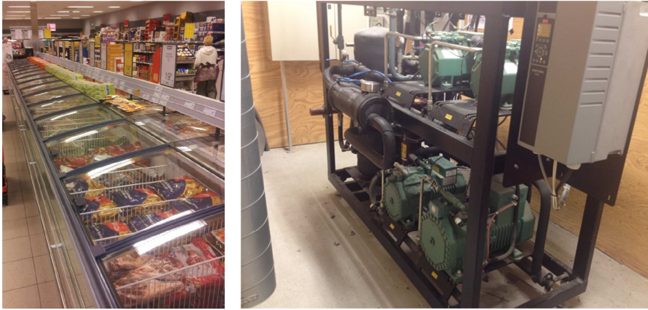
Figure 6.7: Fakta supermarket used for the “PowerCap” experiment (The cold storages and the compressor rack)
