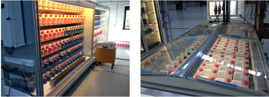
Figure 6.4: A vertical medium temperature and a horizontal low temperature display case at the Danfoss refrigeration laboratory
