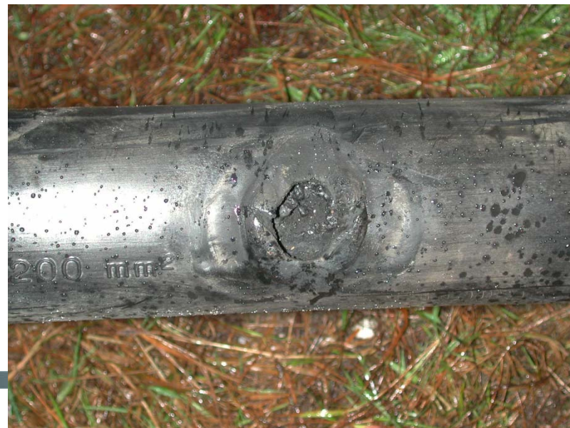
Photo of a single phase cable fault at the onshore part of the Horns Reef 2 170 kV HVAC cable. From PhD Thesis by Christian F. Jensen, 2013.
