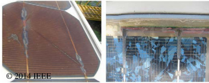
Figure 1.6: Example of corrosion in the busbars and interconnect ribbons observed in different modules (reprinted from [33] with permission from IEEE).
