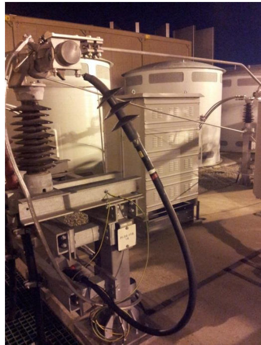
b) Voltage sensor measuring U_{b1} . The filter is connected to the open bus bar (see Figure 5-5a. The phase reactors and converter container can be seen in the background.
