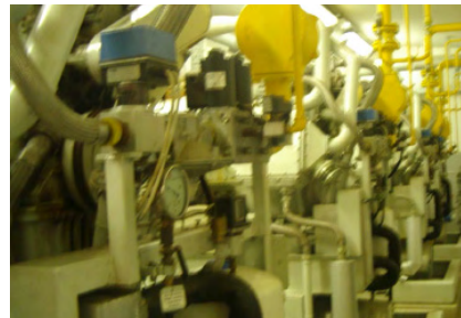
Figure 8 – Biogas engines in Noreikiskes power plant
