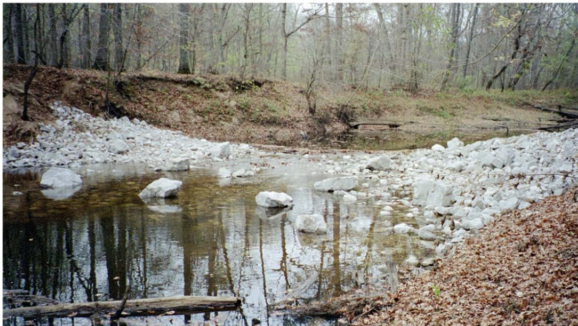
Figure 4.1. The engineering design schematic of a typical riffle weirs and a picture shortly after installation of a weir. Figure and photograph courtesy of John Beardsley of the Illinois State Water Survey.
