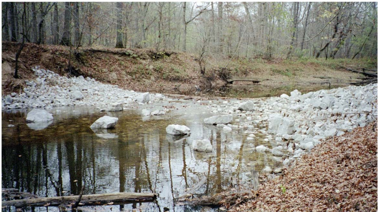
Figure 3.11. The engineering design of the riffle weirs creates a pool upstream of the weir and a tail of shallow rock material to dissipate stream energy.
