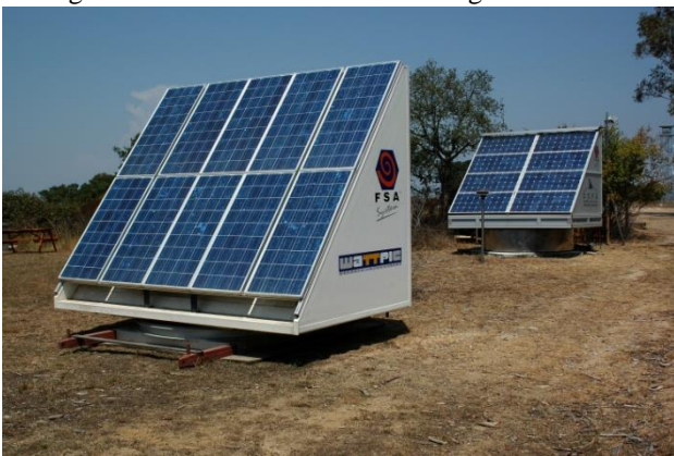
Fig. 4. Photograph of two FSA units installed at Mas Roig.
