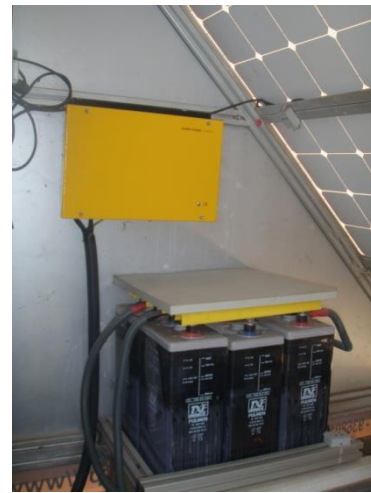
Fig. 5. Detail of the interior view of an FSA, including a set of batteries and its charger.
