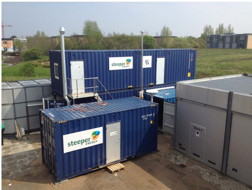
Figure 10: CBS #1 set-up at Aalborg University Campus, Denmark. Container in the front contains the pretreatment unit, the 2 containers in the back contain the process plant in the bottom and the control and utility system in the top.
