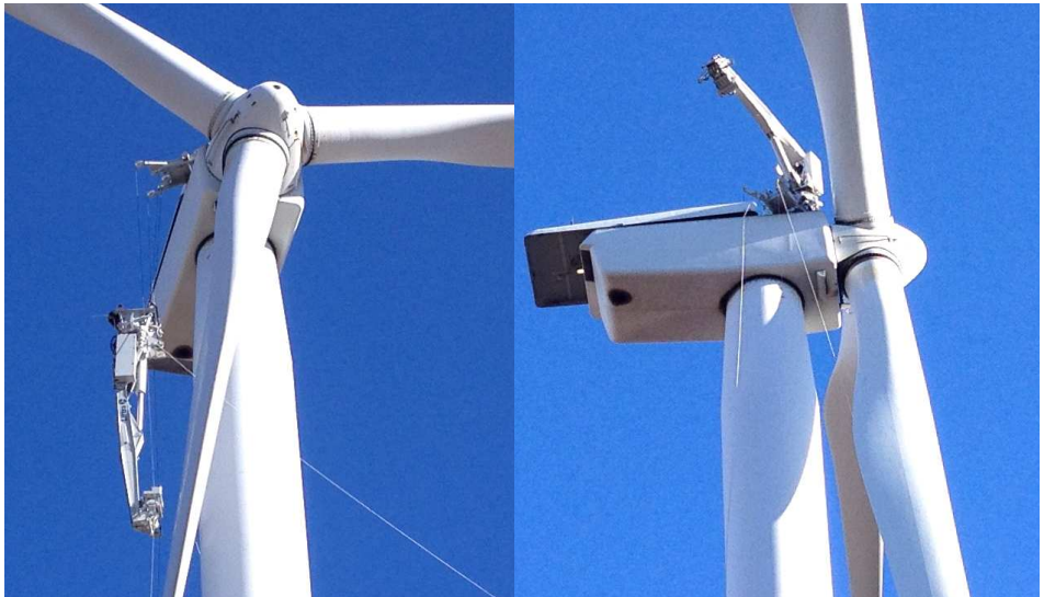
Figure 1.3: A potential motor application is as yaw motor at Liftras self hoisting cranes. Here one is during installation and after the installation on the top of the nacelle of a wind Turbine.
