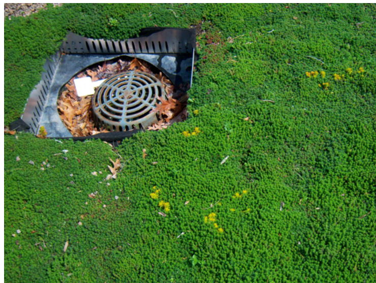
Figure 3. The drain box and sedum establishment on April 12, 2011. Note the thickness of the sedum mat (both pictures by author).
