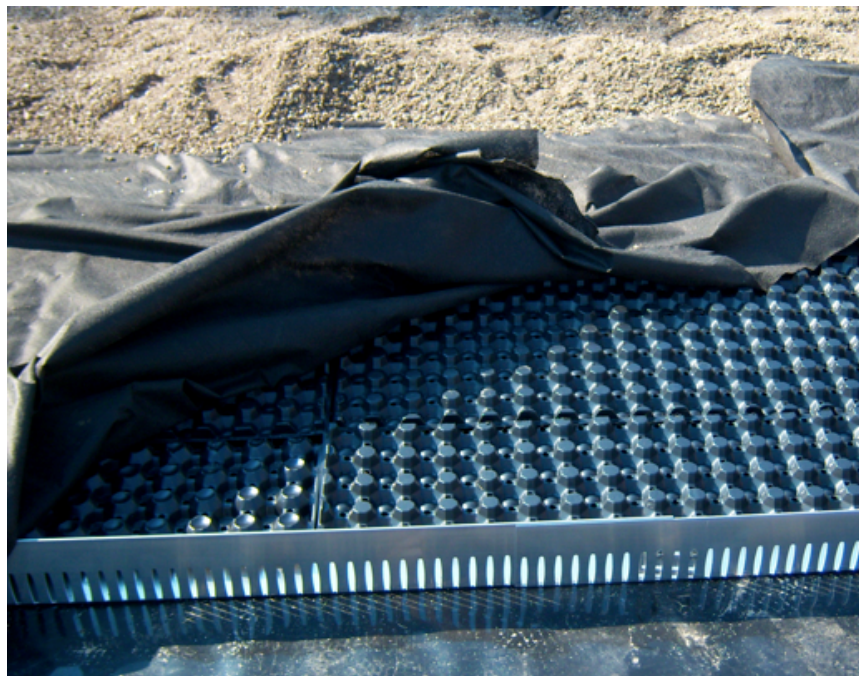
Figure 1. From the bottom layer up; TPO (not shown), moisture retention fabric (not shown), root barrier, drainage layer, filter fabric, and growing substrate. This is contained within aluminum railings (picture by the author).
