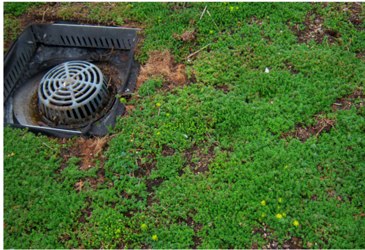
Figure 2. The drain box and sedum establishment on October, 16, 2010.
