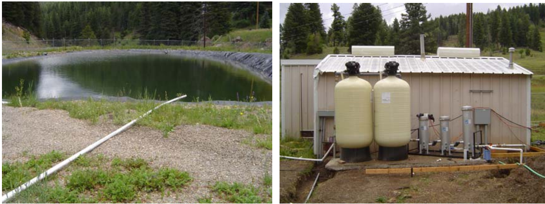
Figure 1. Cloudcroft, NM 1-MG firefighting reservoir and surface water treatment plant.
