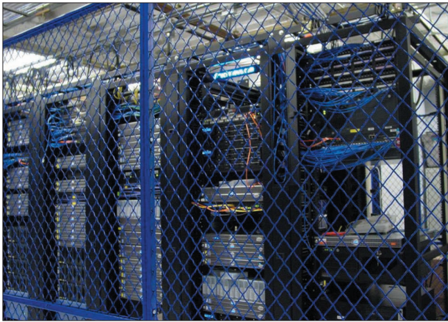
■ Figure 1. Snapshot of row of a typical data center.
