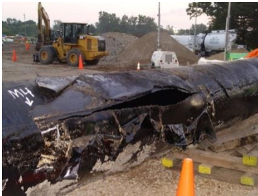
Figure 1. Failure because of high pressure
