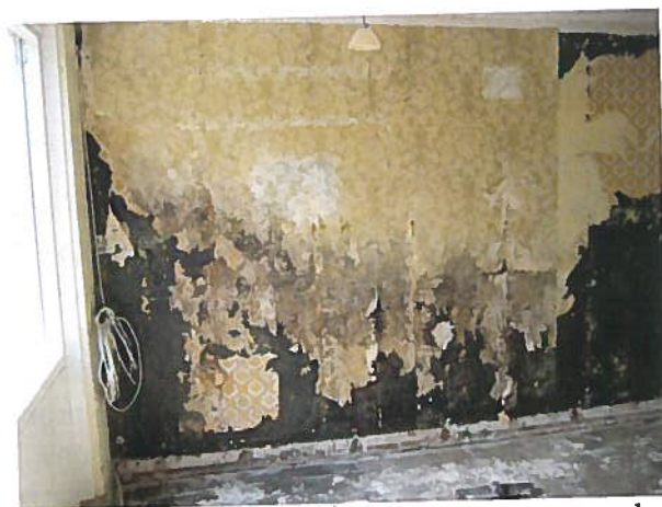
Figure 1. Example of outer wall of 230 mm lightweight concrete where interior insulation has been removed; revealing areas with mould growth.
