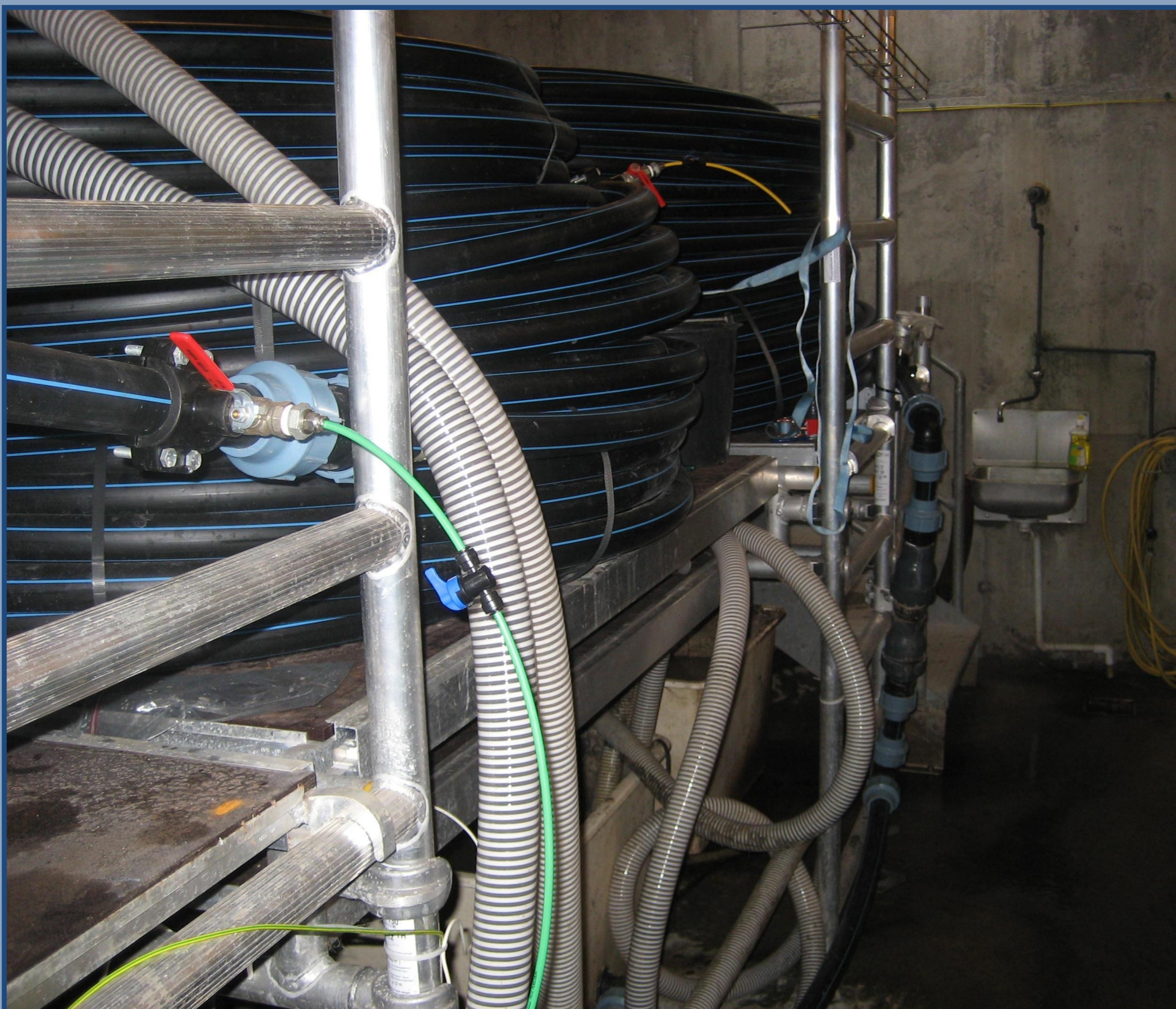
Sewer test facility in Frejlev, Denmark. Under the scaffold the two reservoirs can be seen. From here the waste water is pumped into the 1000 m PE force main (black). The grey hoses forms the loop back to the pump, which is located outside the picture to the bottom left.
