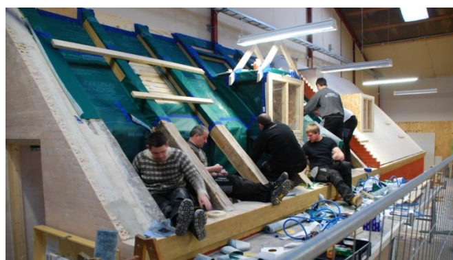
Fig. 9. Continuing education of craftsmen in establishing an airtight vapour barrier in a mock up of an existing roof. Unlike real conditions the roof is placed indoors resulting in far better conditions concerning temperature and lighting.
