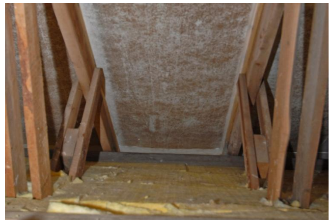
Fig. 4. Rafters with fished joints make it more difficult to install a vapour barrier. In this case the vapour barrier is under the insulation; the mould growth on the roofing underlay indicates that the vapour barrier was not effective.
