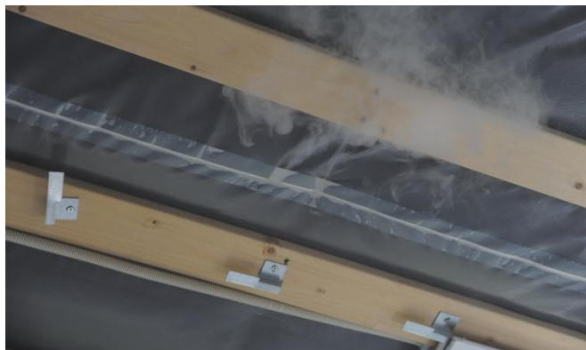
Fig. 5. Taped joint without firm underlay in a new building. The joint cannot be pressed firmly together; as a result small leaks appear where the materials wrinkle. Here illustrated by applying a small overpressure to the construction and adding theatrical fog.
