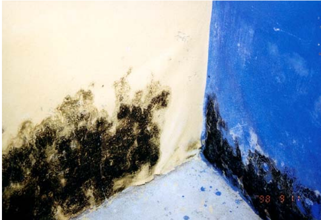
Fig. 2. Growth of mould on wall paper on very moist basement walls due to considerable ingress of moisture through the walls and the connection between floor and wall (often very vulnerable).
