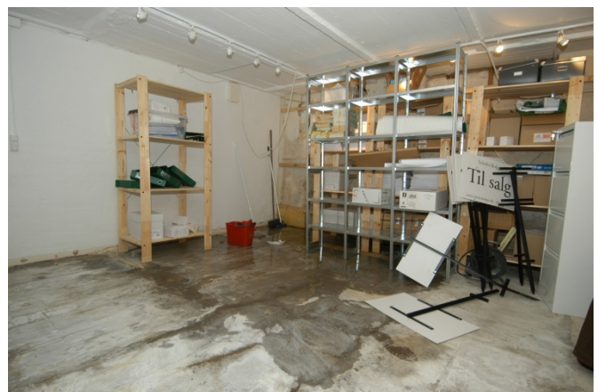
Fig. 1. Penetration of water through cracks in a basement wall in periods with heavy rain – cracks were due to bad workmanship. The moist conditions are very unfortunate as the (new) owner uses the room for storage of paper.
