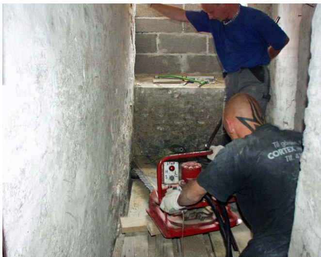
Fig. 6. Large chain saw with diamond tipped teeth. Found to be the best option for making through joints in basement walls.
