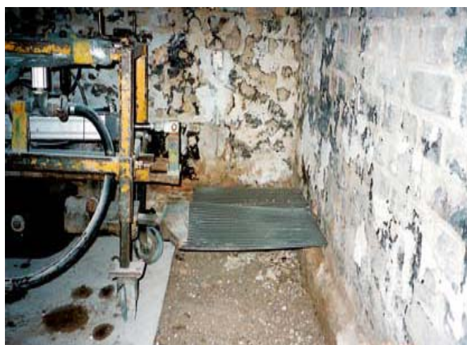
Fig. 4. Installation by vibration of a corrugated steel plate in a through joint in a masonry wall. The machinery is large and demands a lot of space in front of the wall. If the basement floor is removed it is an advantage to install from the inside.
