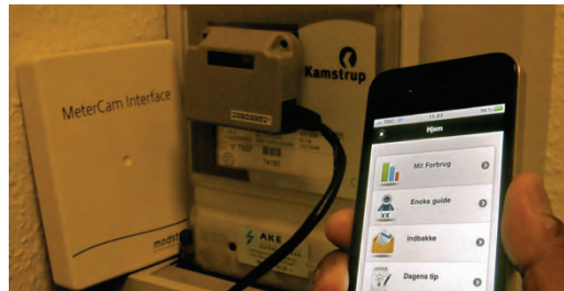
Figure 4. Modstrøm’s Automatic Meter Reader mounted on the readout of an old mechanical meter
