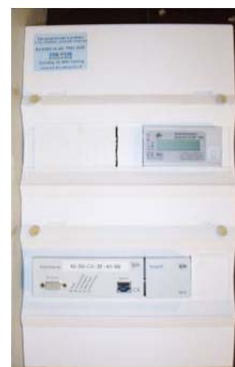
Figure B.0.5: Electricity meter.
